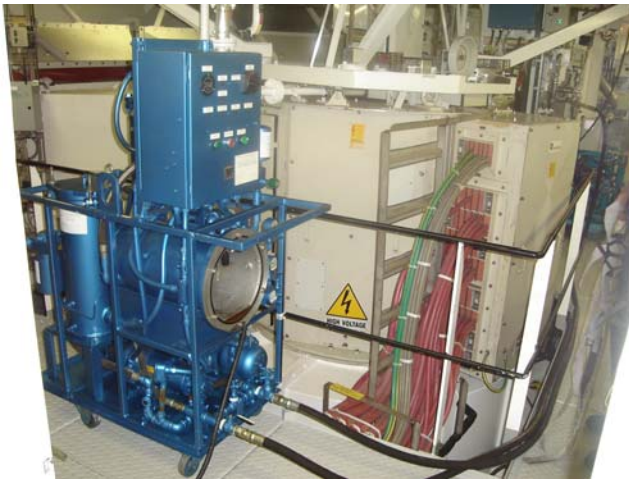
3 GPM VDOPS Operating on an Azi-Pod Lube System
