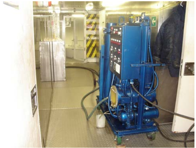
5 GPM VDOPS Operating on an Fixed-Pod Lube System
