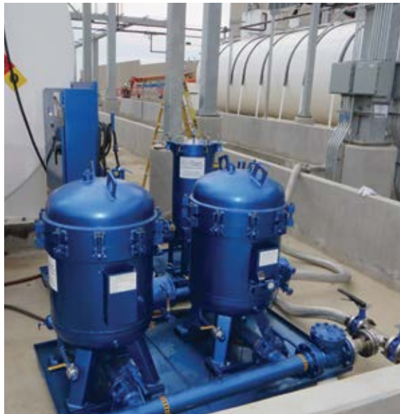
High Velocity Fuel Oil Flush of a backup generator fuel system at a data facility
